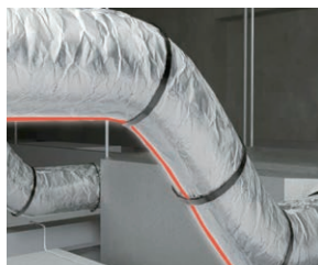
Attached to piping
